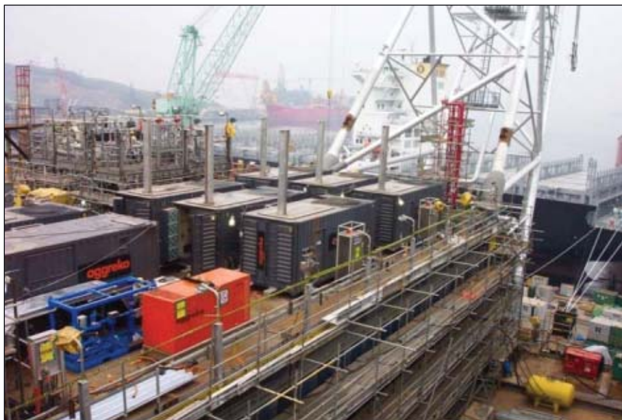
Construction and commissioning of the Sakhalin-2 LUN-A platform required temporary power and safety packages (Fig. 1). Photo from Aggreko.
